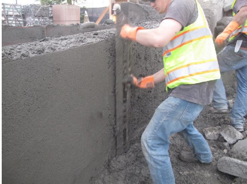
Fig.8 Trimming shotcrete to shooting wires in straight wall with cutting screed (rod)
